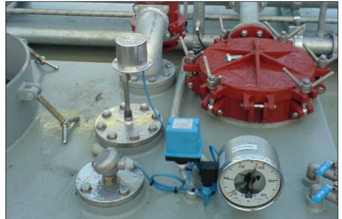
Fig. 1: Onsite display of the Level Plus® Transmitter (source: ITU).
